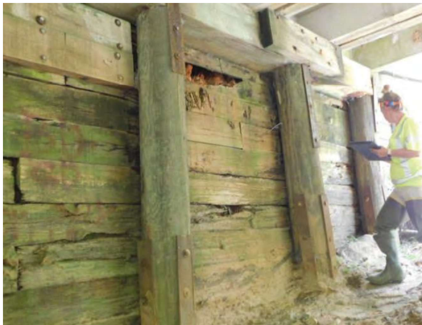
BREAST WALL BOARDS ABUTMENT 2 DECAYED
