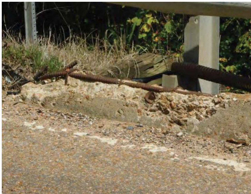
LEFT SIDE CURB SPAN 1 SPALLED TO STEEL
