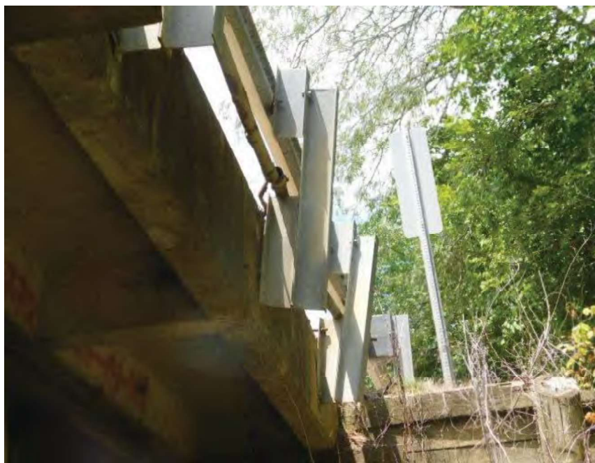
LEFT SIDE SPAN 1 RAIL BROKEN LOOSE
