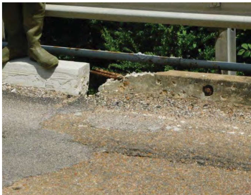
LEFT SIDE CURB SPAN 3 SPALLED TO STEEL
