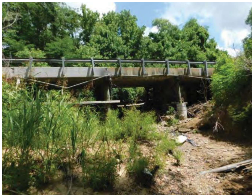
RIGHT SIDE OUTLET END
